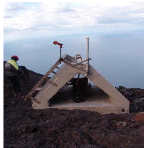
Leica Geosystems equipment in a concrete cage
