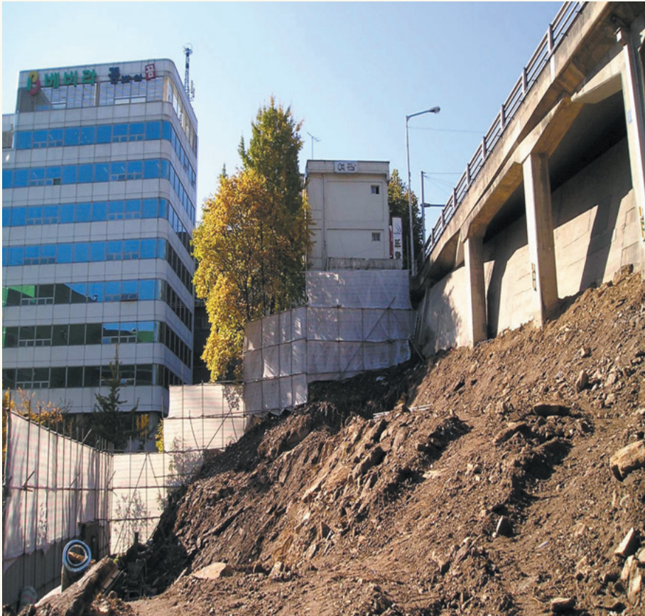
High-definition surveys are used for monitoring structures near excavations. Image Courtesy: Dasan Engineering
