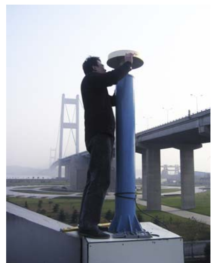
Mr. Li of Leica Geosystems partner EuroAsia installing a GPS monitoring station
