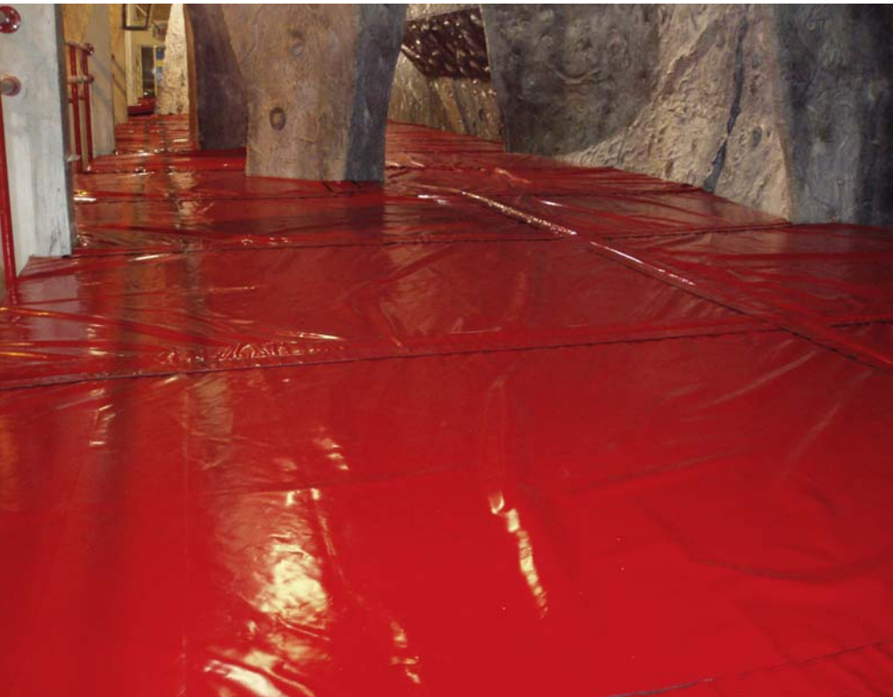
The finished flooring mat. The mat had to be cut to fit round complex obstacles.
