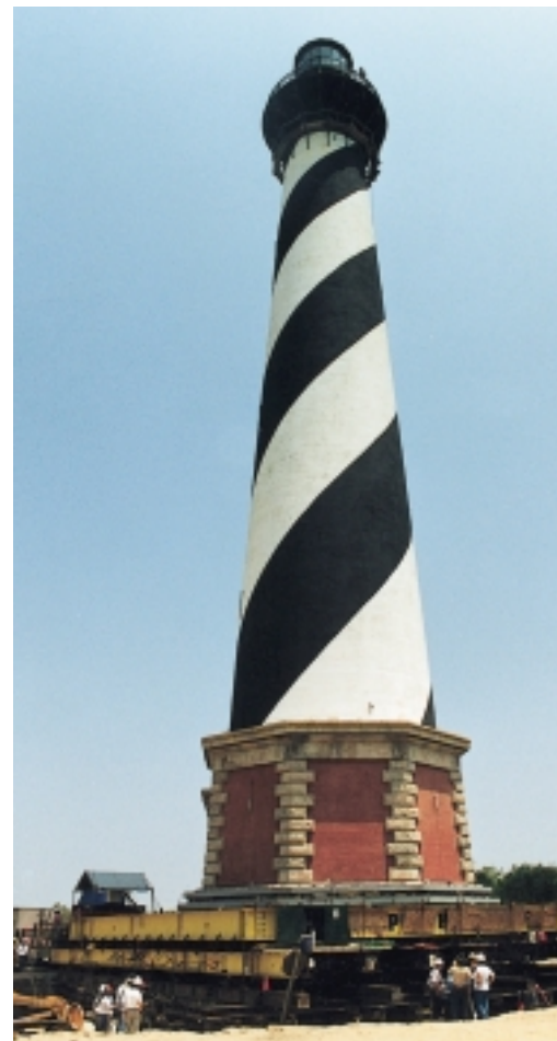
The Hatteras lighthouse on its steel base and seven track rails as it nears the new location.
